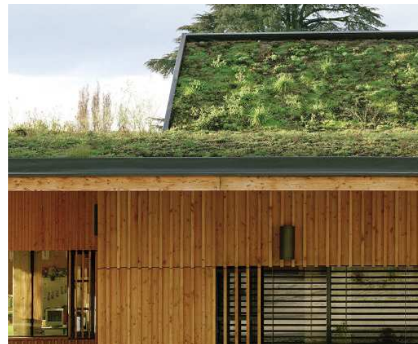
Example of a roof planted with diverse species native to the wooded area.
